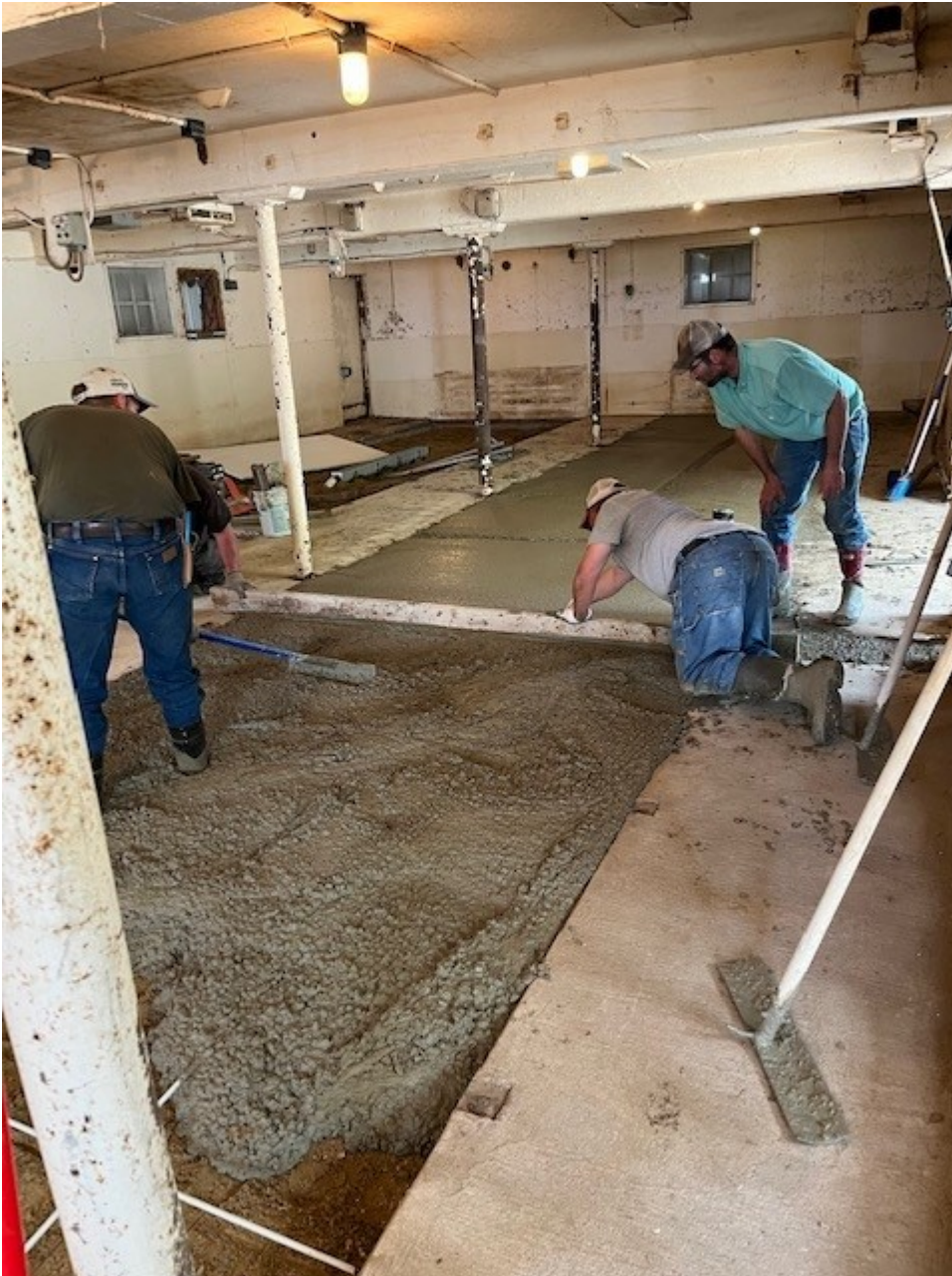
Kittleson Brothers have begun laying concrete for the foundation of the new walk-in cooler and potato sizer purchased with Choose Iowa grant funds.
