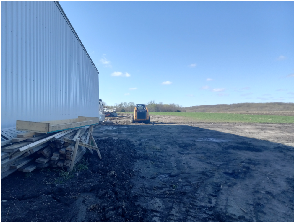
Before the shipping containers could arrive, the land had to be prepared.
