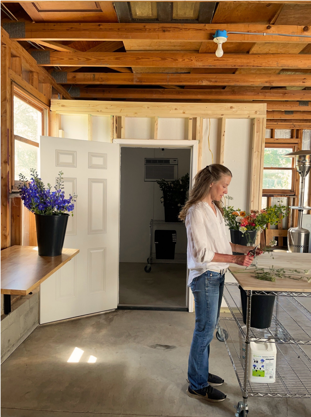
The Choose Iowa project is underway with the construction of the new processing area and walk-in cooler pictured above.
