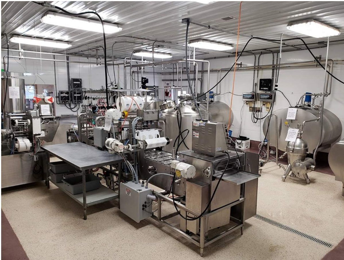
To produce frozen yogurt, Country View Dairy must have a large production room with lots of equipment.
